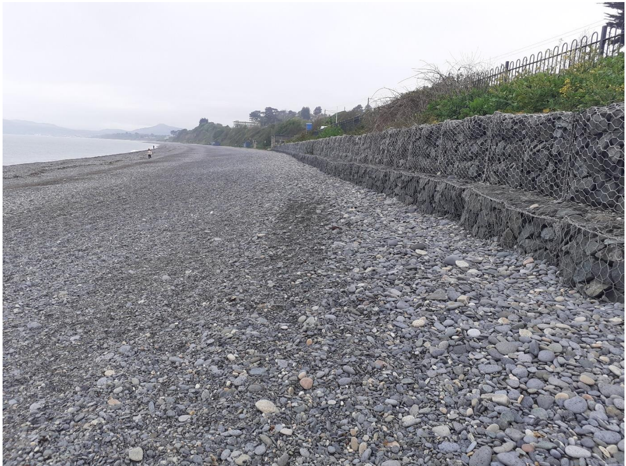
Figure 3-2: Shingle banks (CB1) developing above the high tide line along the base of the gabion baskets
