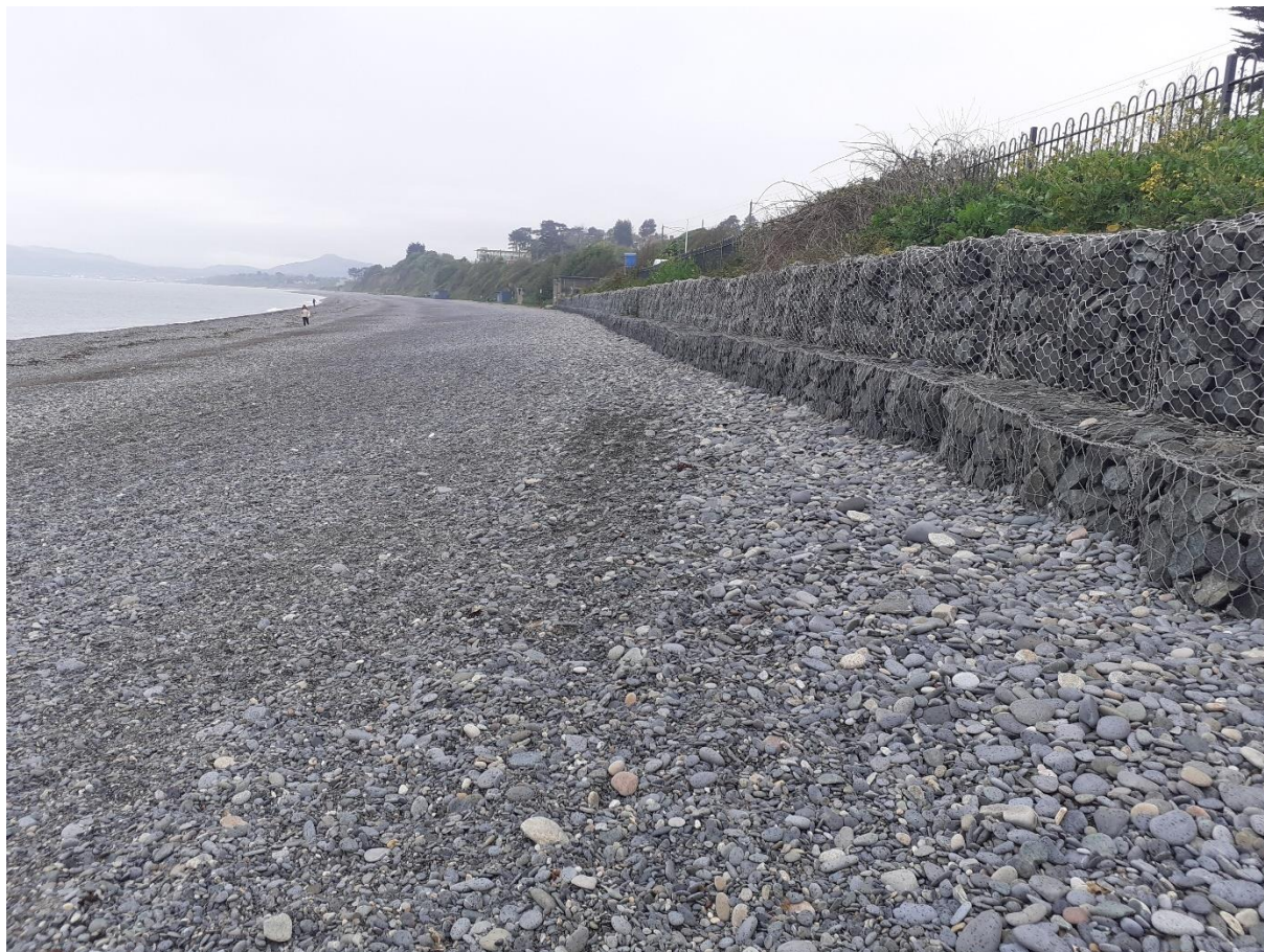
Figure 4-7: Shingle banks (CB1) developing above the high tide line along the base of the gabion baskets
