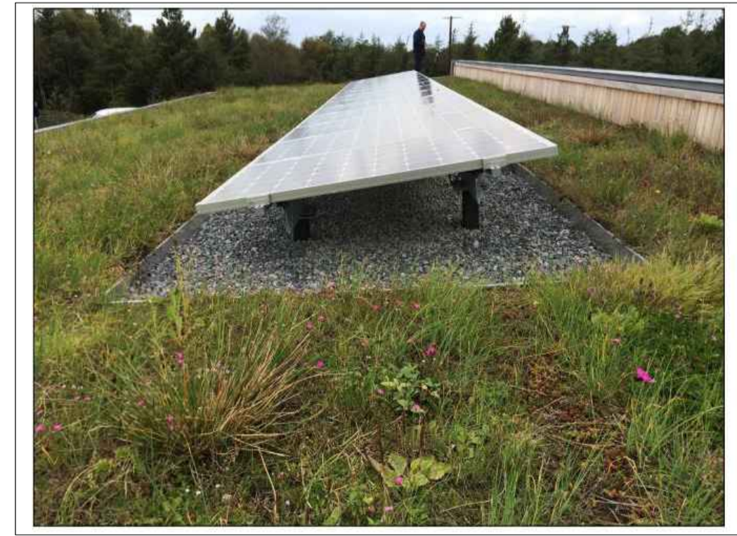
PV PANEL ON GREEN ROOF Scale at A1 NTS Scale at A3 NTS
