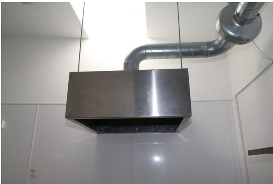
Plate 65: Extract system in scullery
