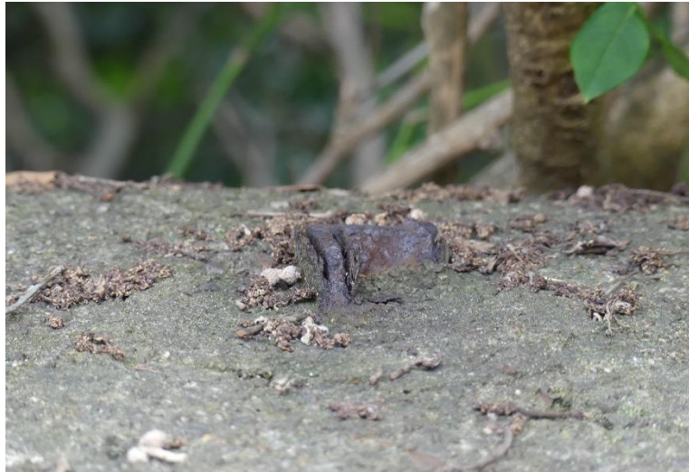
8 Presence of embedded metal fixtures in wall capping
