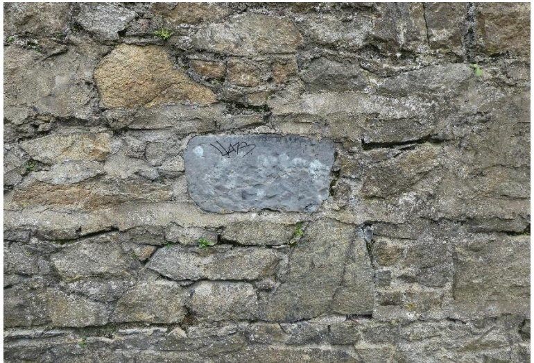
3 Presence of occasional limestone rubble elements possibly introduced during previous repairs
