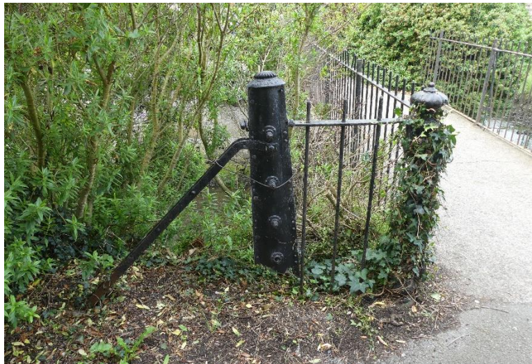
5 Looking west with original metal post on the left and partial metal detailing supported with strut
