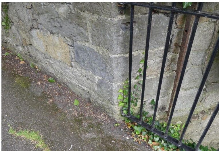
1 Limestone Quoin Details and non-original railing
