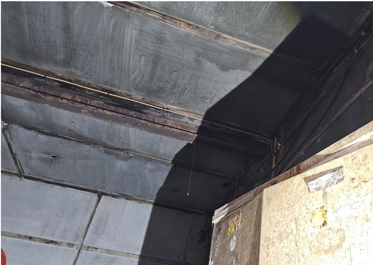
Photo 8. Internal ceiling of extension (Ground floor) – Serious corrosion to steel beam evident
