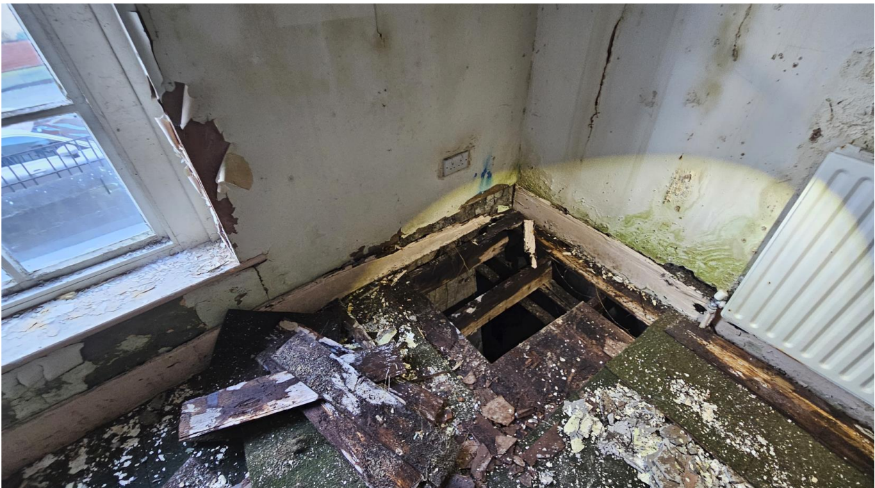
Photo 6. Internal floor of extension (First floor – front). Close up of hole in floor
