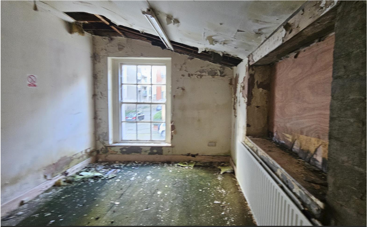
Photo 5. Internal floor of extension (First floor – front). Water damage has caused hole in floor
