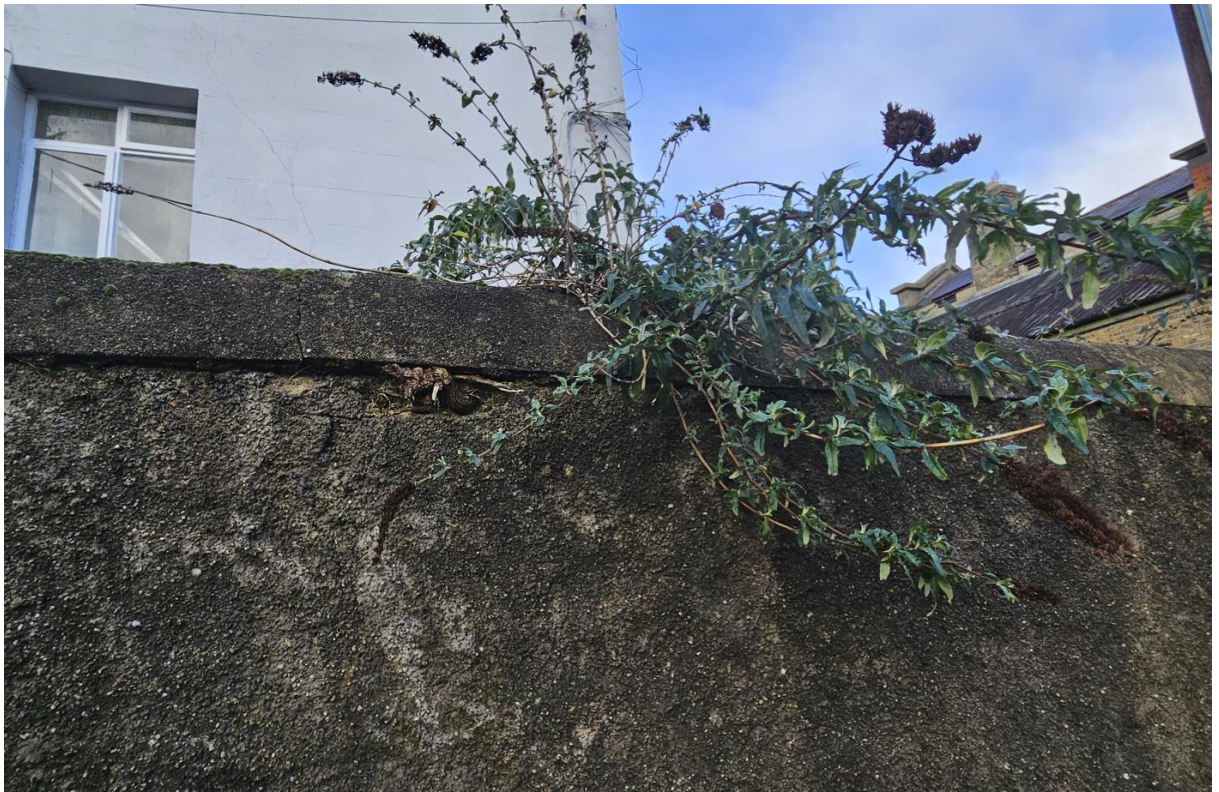
Image 11. Vegetation growth in boundary wall
