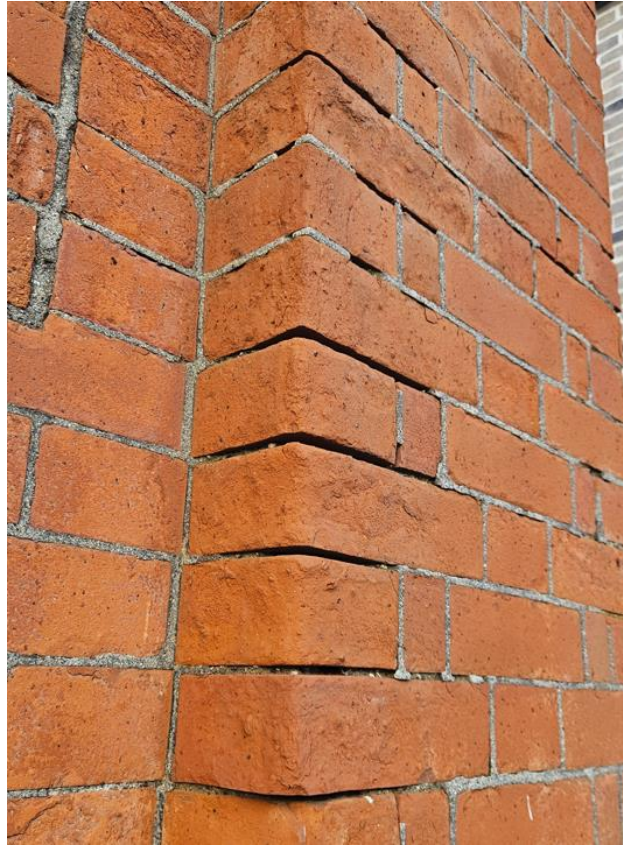
Image 23. Wash House building. Example of washed-out mortar joints
