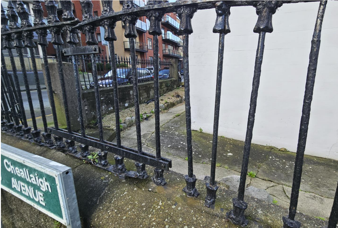
Image 9. Close up view of damaged railings requiring repair
