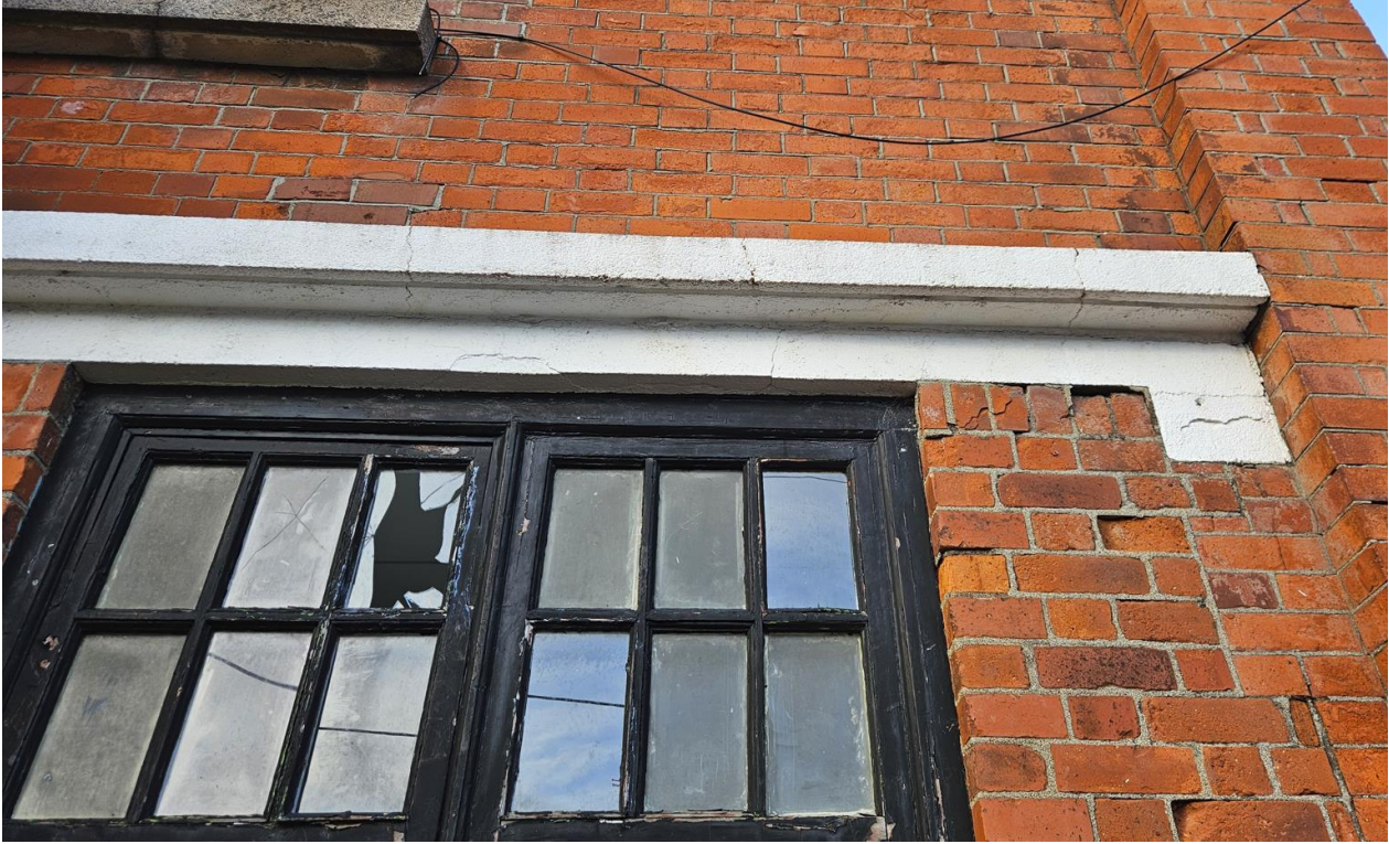
Image 27. Wash House building. Example of cracked/ debonded concrete window cill
