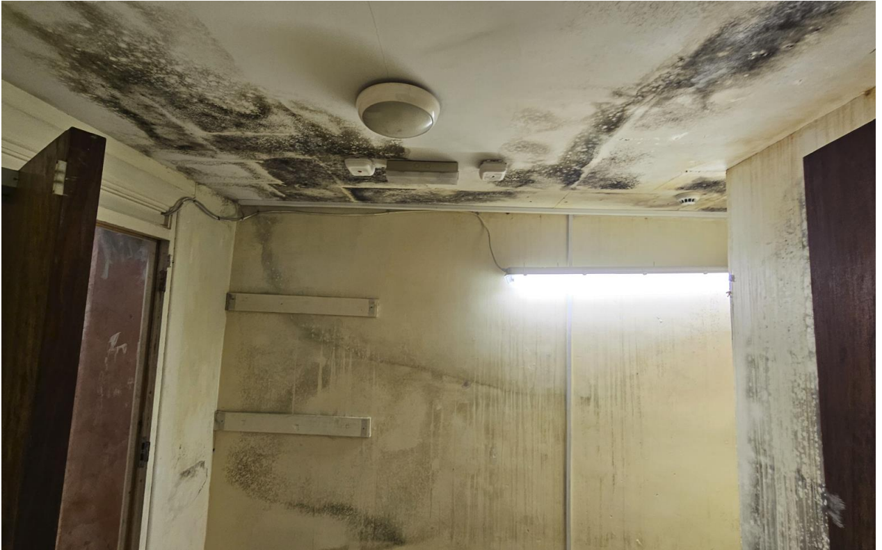
Image 15. Internal view of lower ground floor corridor. Signs of mould, algae, wet and water staining from roof leak three levels above.
