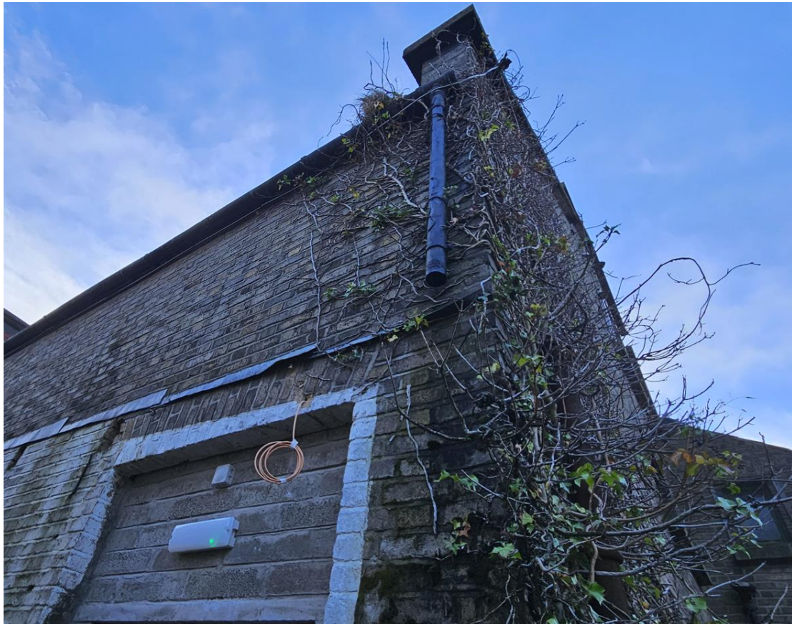
Image 28. Wash House building. Missing section of down pipe and vegetation growth causing damp issues internally
