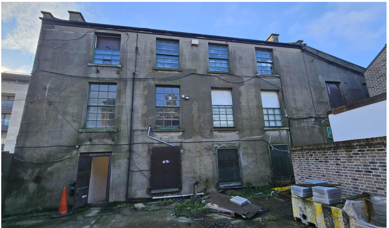
Image 4. View of side wall of No. 9 Georges Place (north-east facing). Note the missing down pipes, excessive redundant cables, various cracks to wall, algae staining to render
