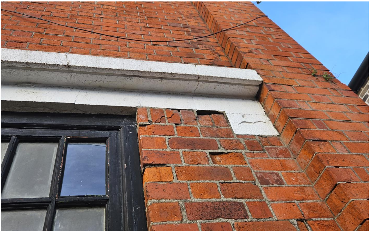
Image 30. Wash House building. Missing and damaged brick faces
