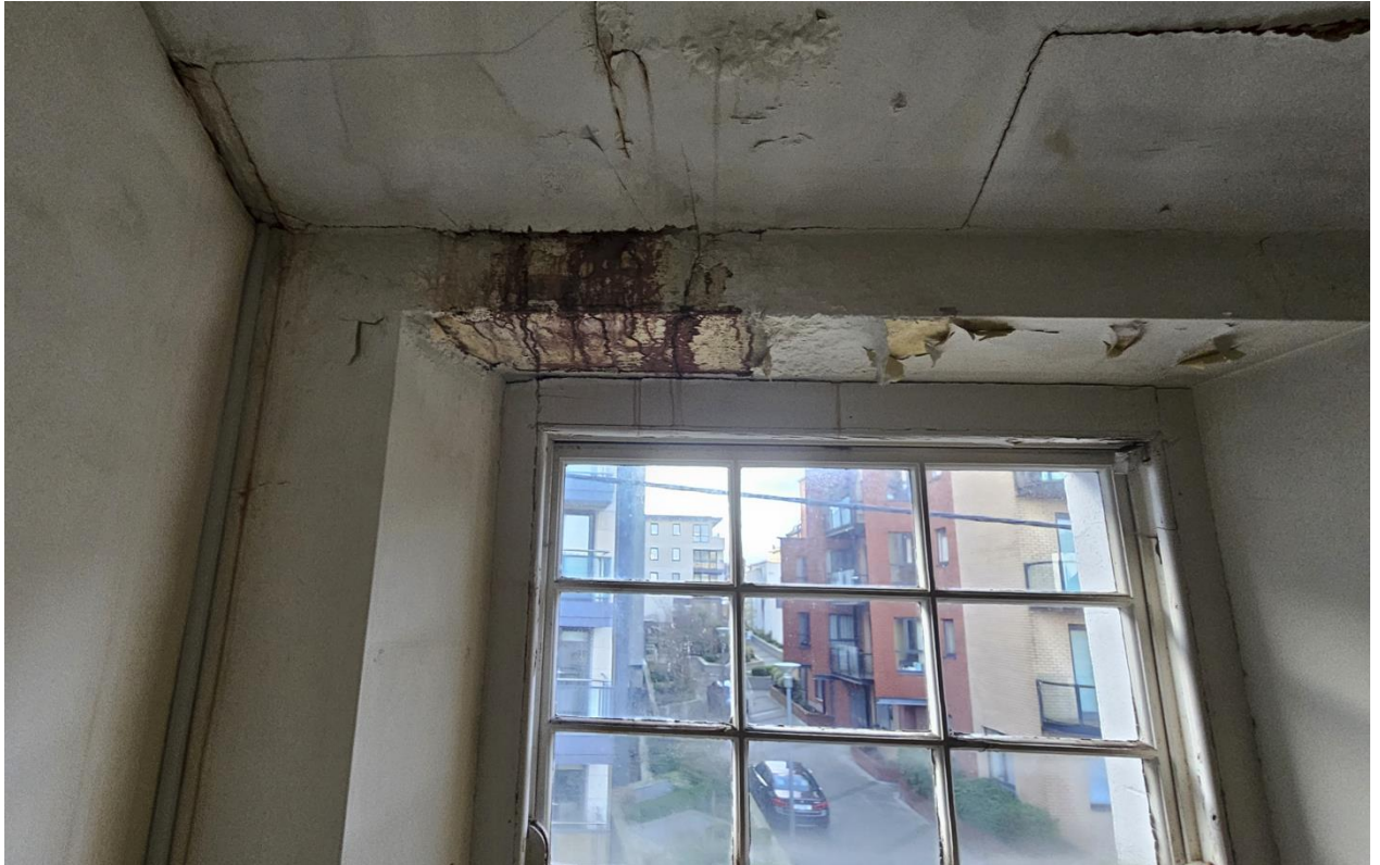
Image 21. First floor gable wall, evidence of damaged window lintel
