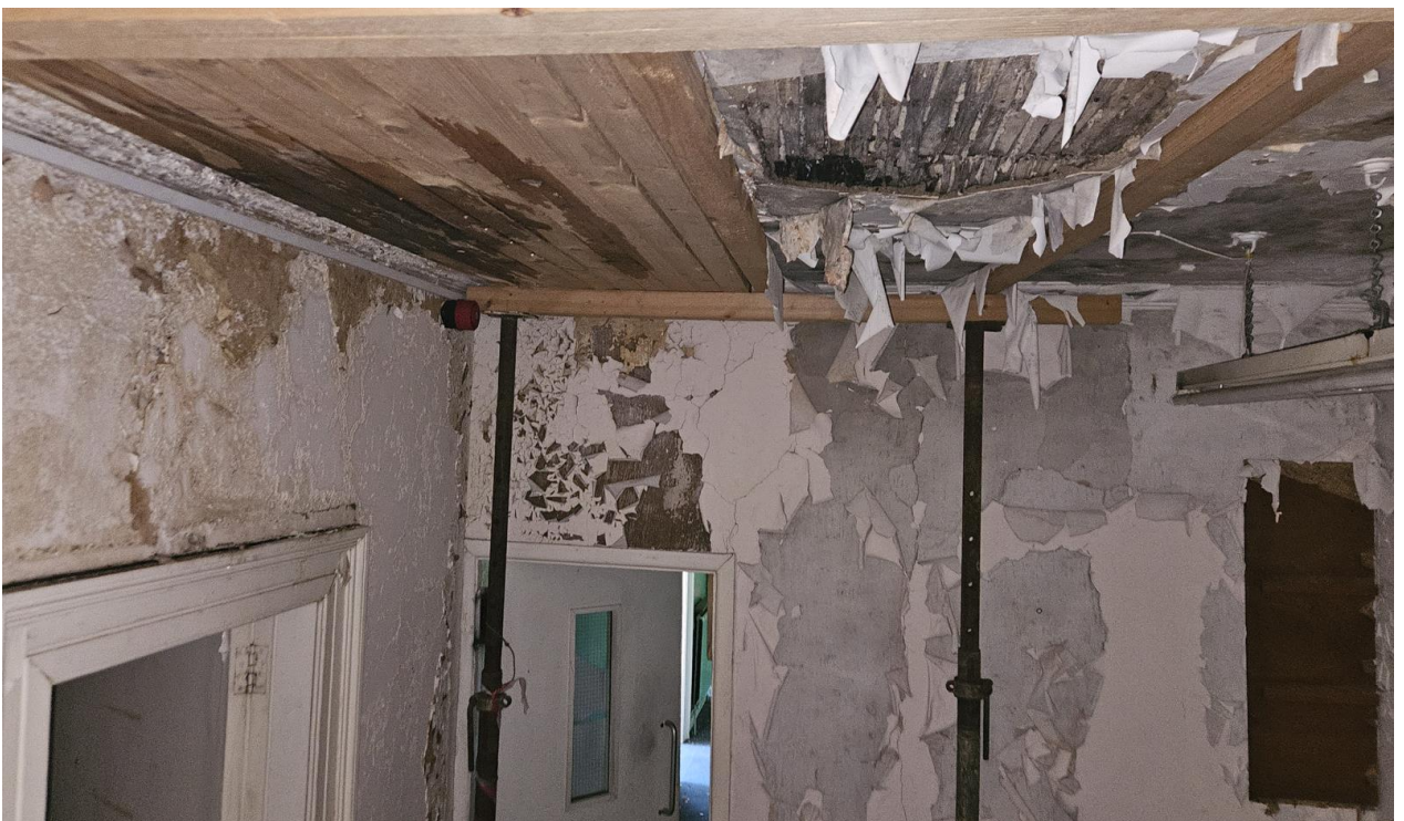
Image 16. Upper ground floor corridor ceiling has failed and is being support by temporary props and a timber deck.
