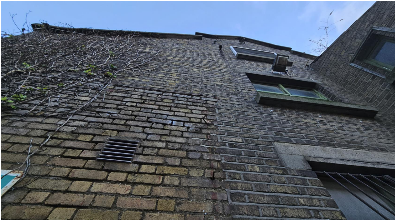
Image 8. View of rear wall of the former Wash House building (north – west facing)
