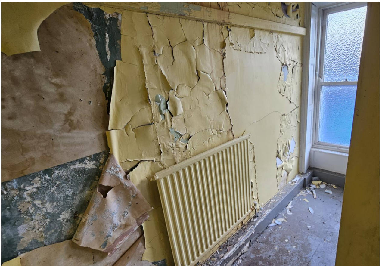
Image 20. First floor gable toilet room. Damage to plaster to internal wall
