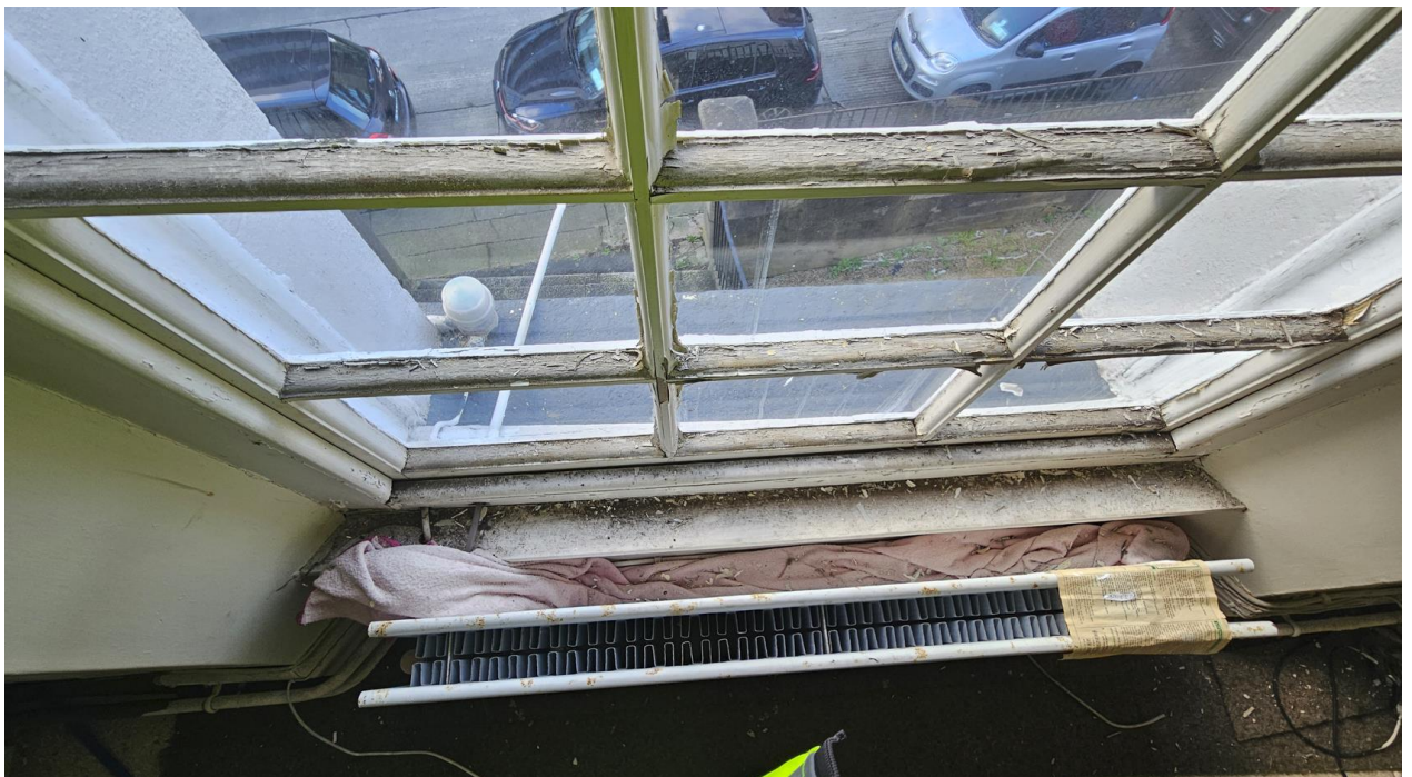
Image 22. Typical condition of timber windows. Requires refurbishment.
