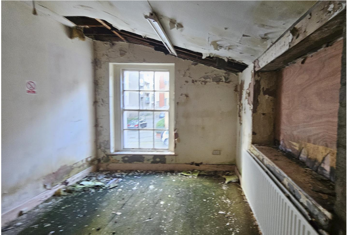
Image 17. Upper ground floor, side extension, northwest room. Roof, floor and walls damage caused by water ingress
