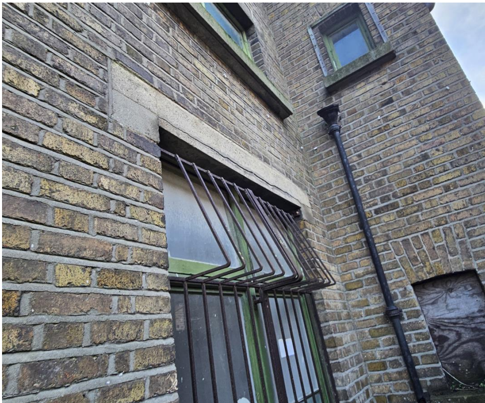
Image 26. Wash House building. Example of cracked/ debonded concrete window cill
