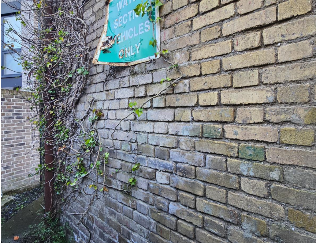
Image 25. Wash House building. Example of washed-out mortar joints
