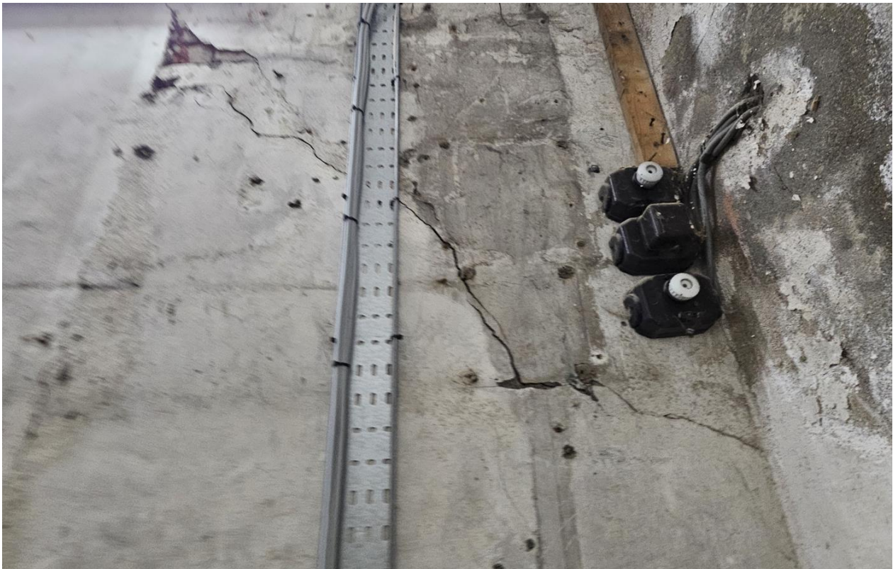
Image 24. Wash House building. Example of cracking to internal walls requiring repair
