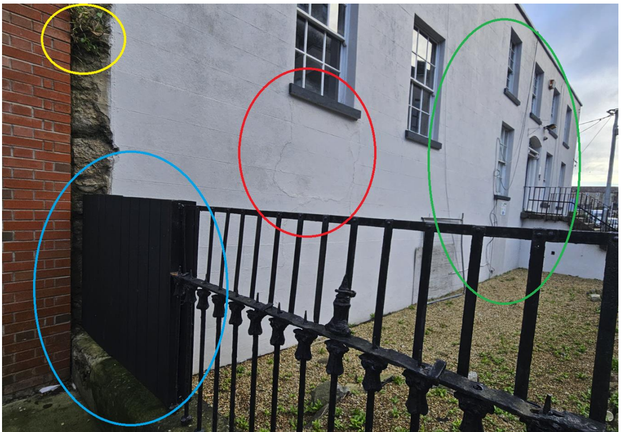
Image 12. Front elevation with vegetation growing from wall (yellow circle), cracking to wall (red circle), redundant cables hanging from building (green circle) and missing section of railing (blue circle)
