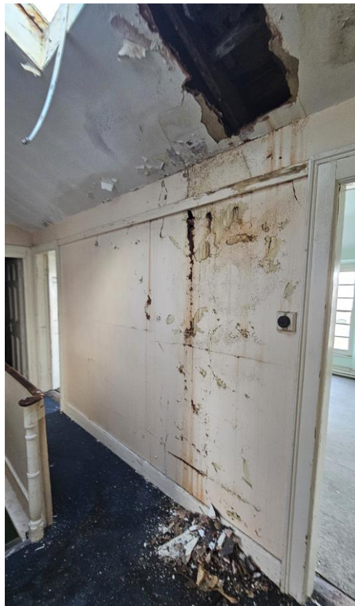
Image 18. First floor corridor spine wall, damage caused by roof leak
