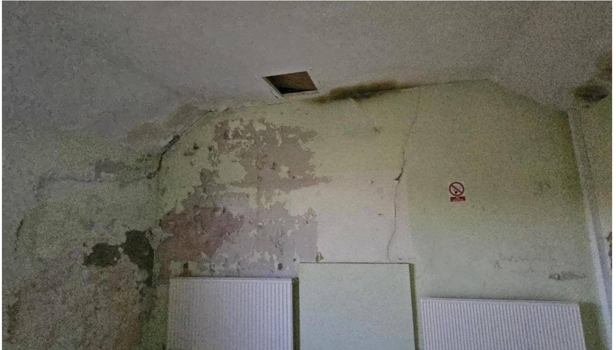
Image 19. First floor rear room masonry dividing wall. Damage caused by damp ingress and crack visible requiring repair
