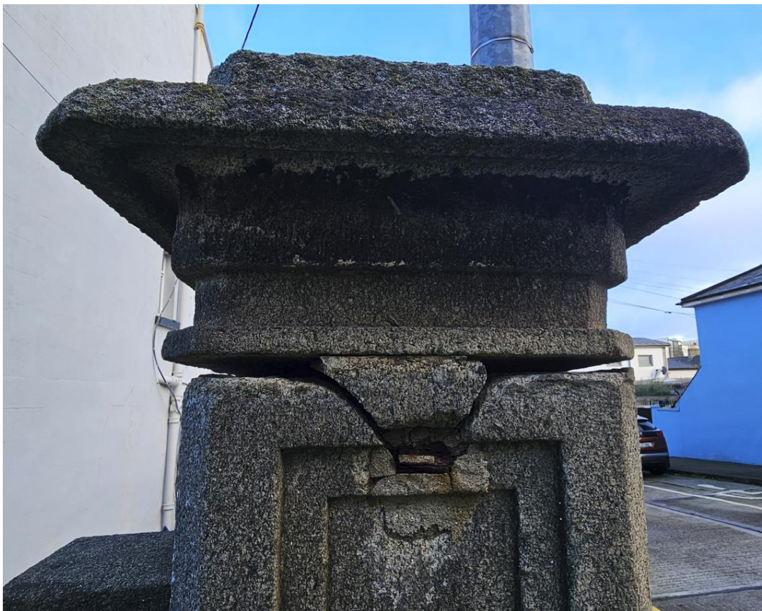
Image 10. Close up view of boundary corner stone pillar. Metal insert has corroded causing expansion and cracking and raising of stone cap
