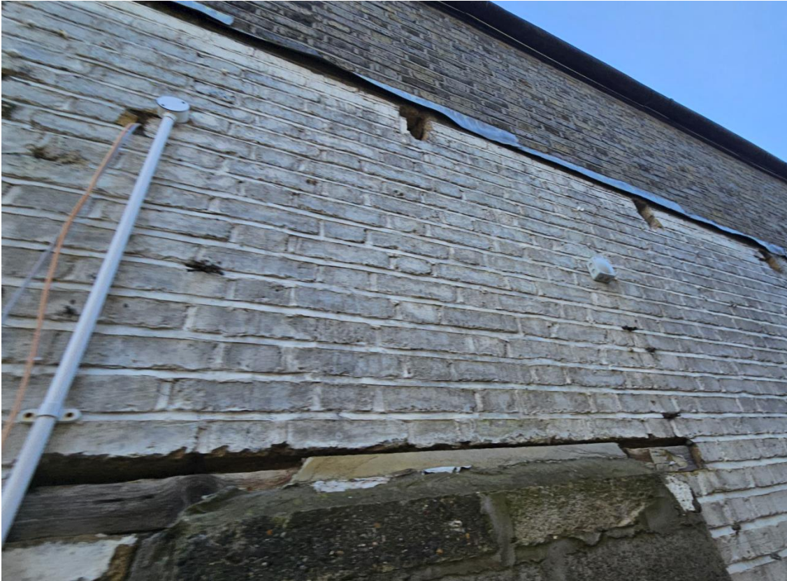
Image 29. Wash House building. Exposed timber lintels and high level holes in external wall.
