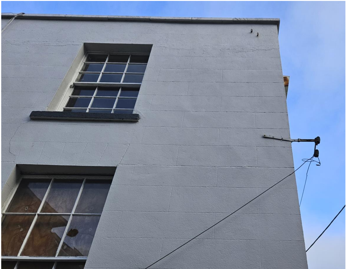
Image 14. External view of front elevation. Remove loose redundant cables and associated metals supports.
