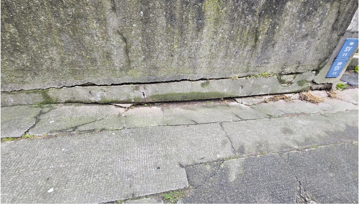
Image 13. Close up view of external front boundary wall. Cracking to base requires investigation
