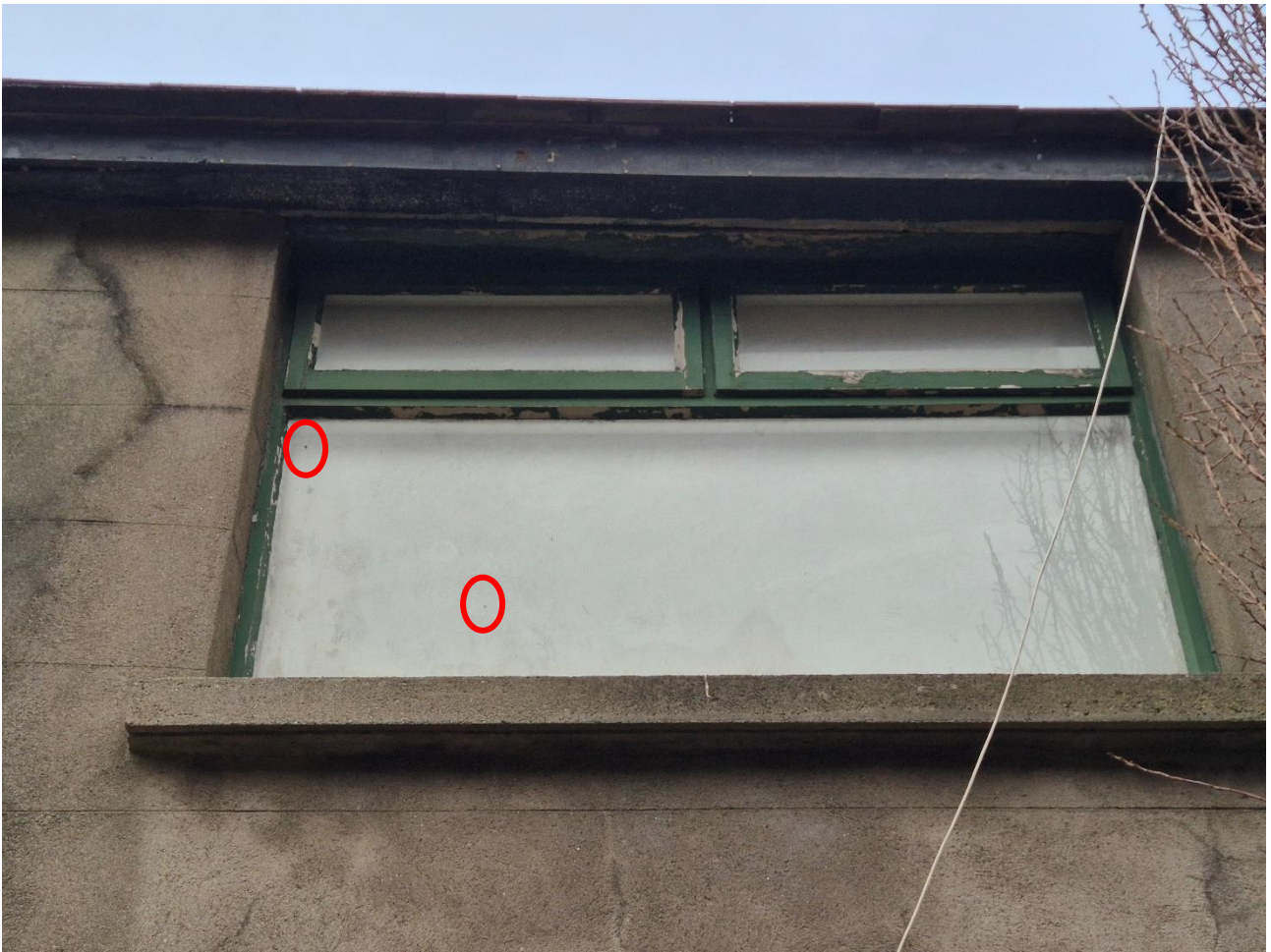
Plate 1: Bat droppings on window pane (external), No. 9 Georges Place, Kellys Avenue, Dún Laoghaire, Co. Dublin.
