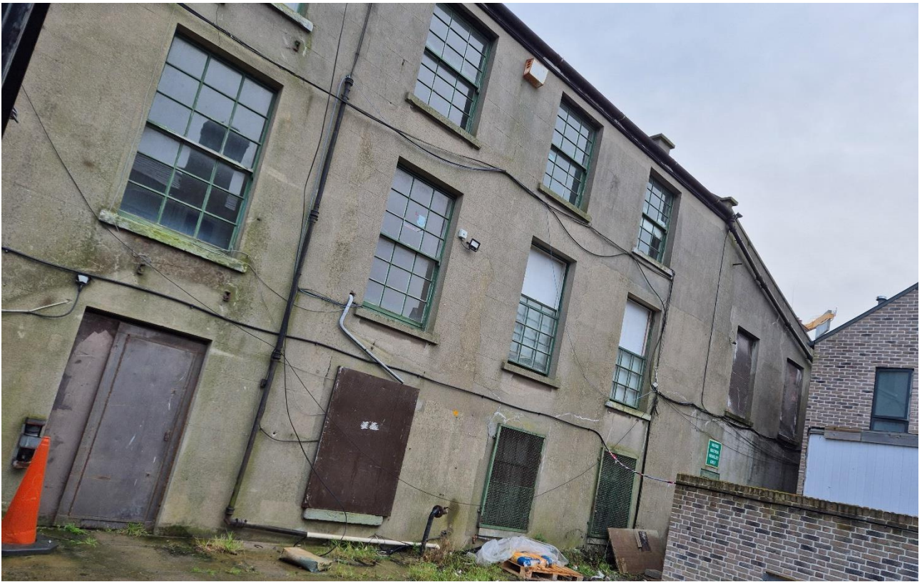
Plate 3: Rear view of No. 9 Georges Place, Kellys Avenue, Dún Laoghaire, Co. Dublin.
