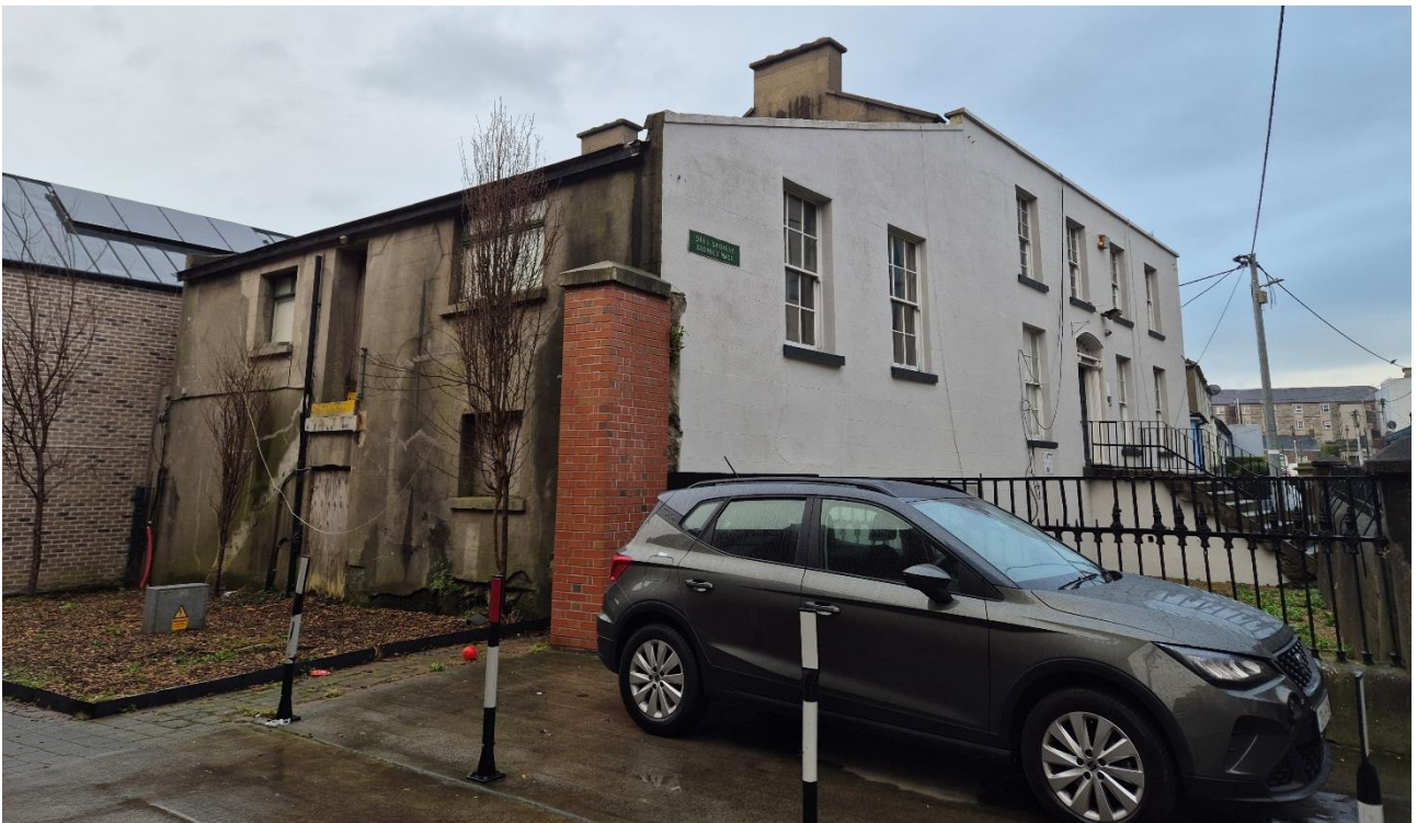
Plate 2: Gable and Front view of No. 9 Georges Place, Kellys Avenue, Dún Laoghaire, Co. Dublin.
