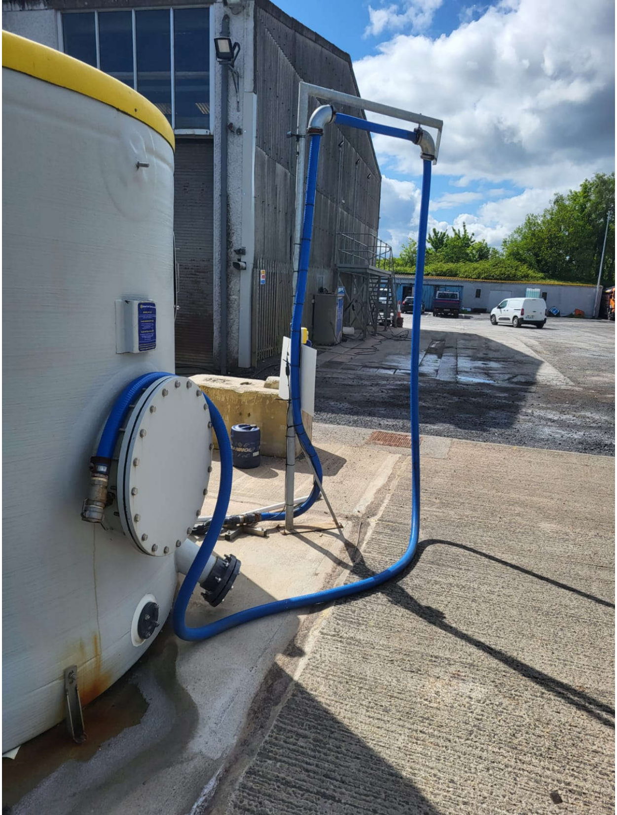
Brine Batching Facility – Mullingar, Co. Westmeath – Truck Filling Point
