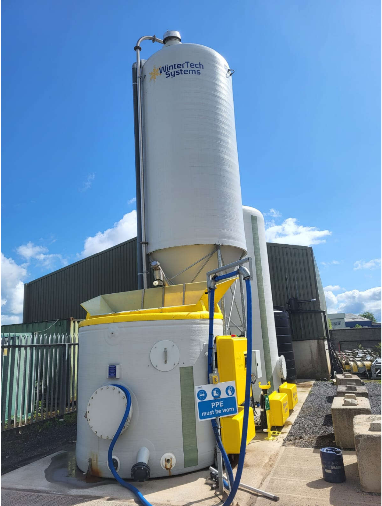
Brine Batching Facility – Mullingar, Co. Westmeath – Brine Mixing Tank and White Salt Silo
