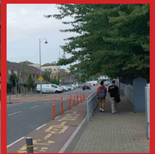
Flexible bollards in poor condition
