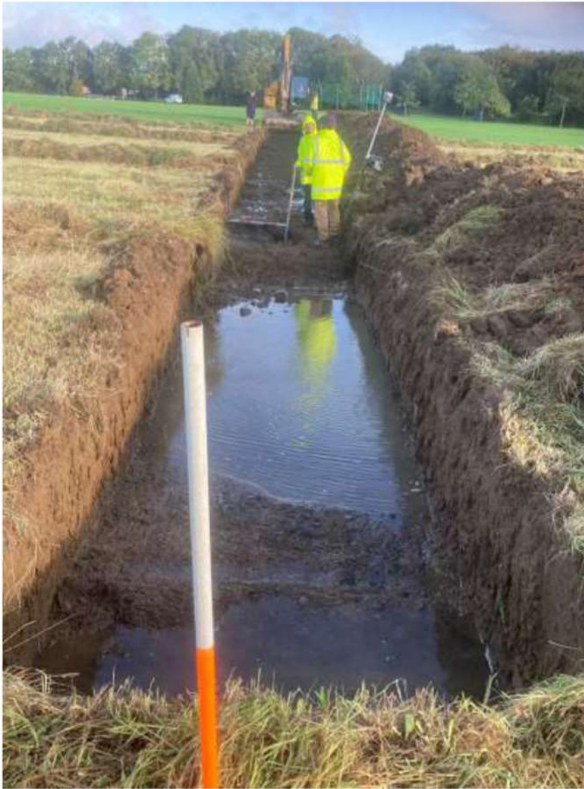
Plate 5: Trench 1 with water ingress, facing north
