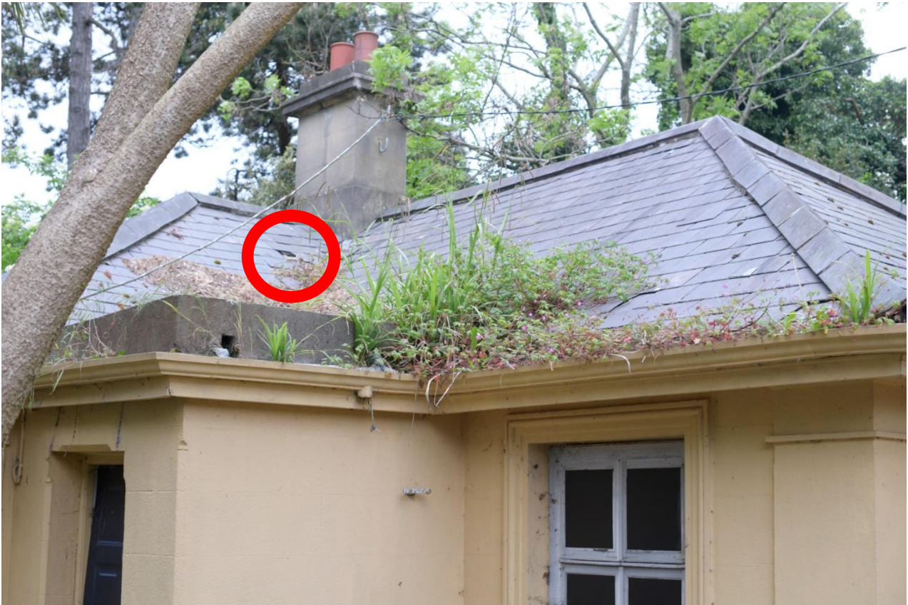
Plate 1. Missing slate on roof.
