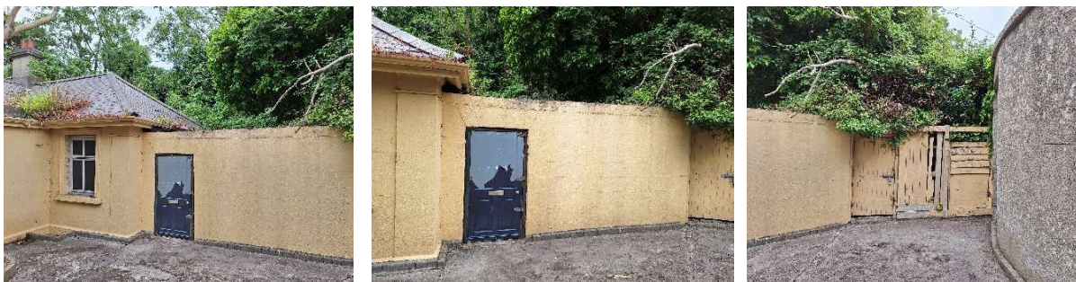
Fig. 11, 12 & 13 Window to recessed bay of gate lodge, modern flat-roofed extension to north-east of gate lodge, gate and fence between extension and boundary wall.
