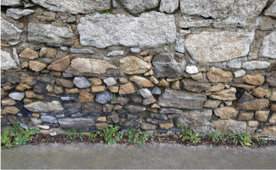
Fig. 48. Sample view of existing random rubble wall to Dundrum Road
