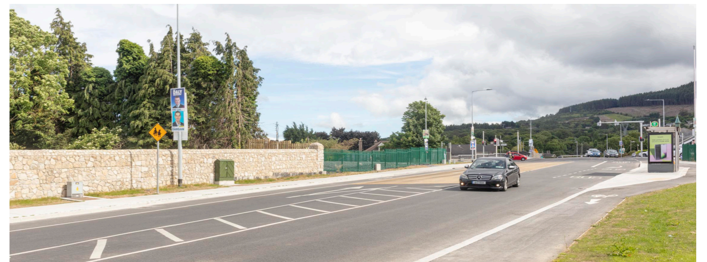
Image 18: 2024- Roadworks complete, junction widened with new footpaths, lighting etc. New perimeter fencing installed
