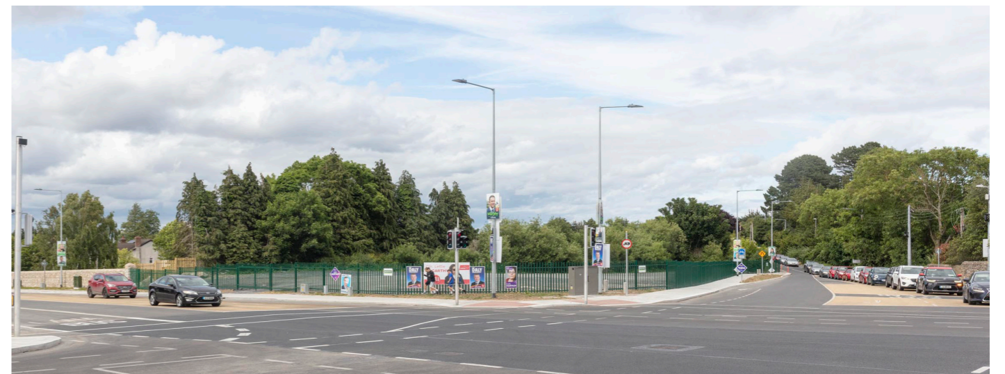
Image 14: 2024- Roadworks complete, junction widened with new footpaths, lighting etc. New perimeter fencing installed
