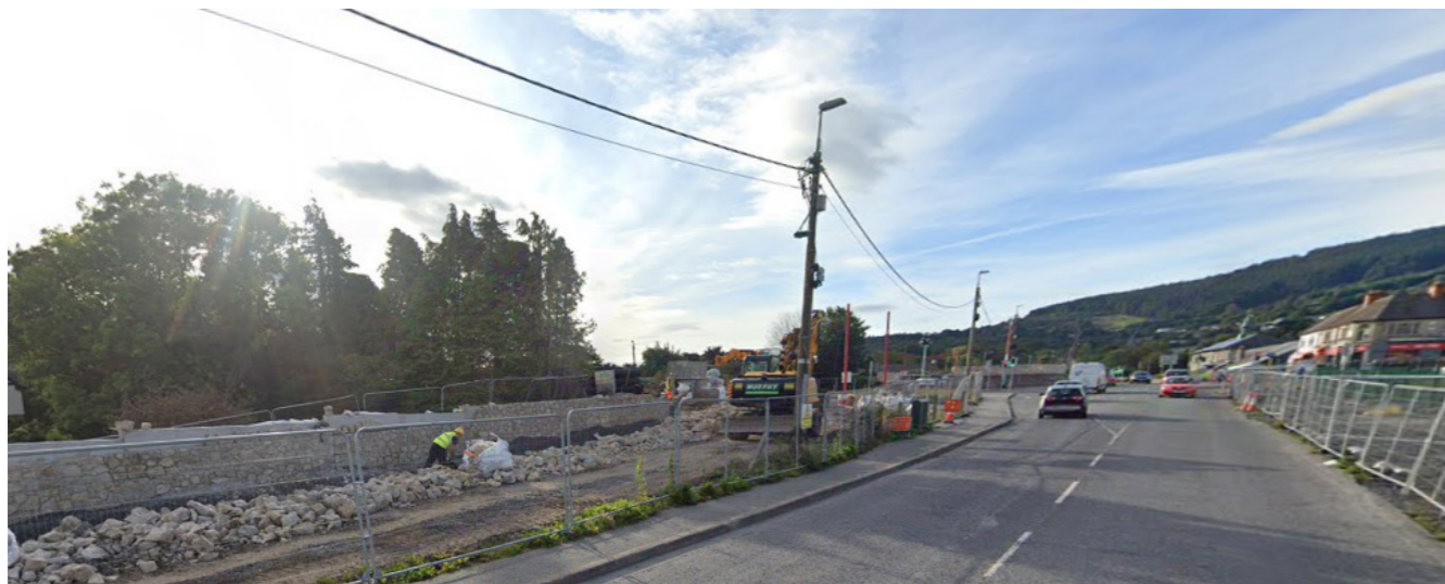
Image 17: 2022- Much of the vegetation removed. The site in use as a compound for the roadworks. Stone clad wall under construction illustrates the difference in road width between existing and proposed.
